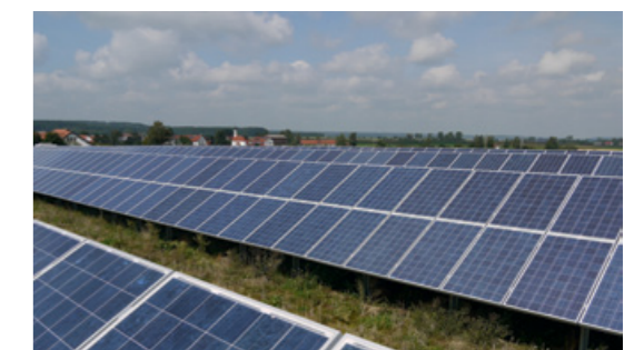
265 kWp, ground-mounted installation, commissioning: 2010
