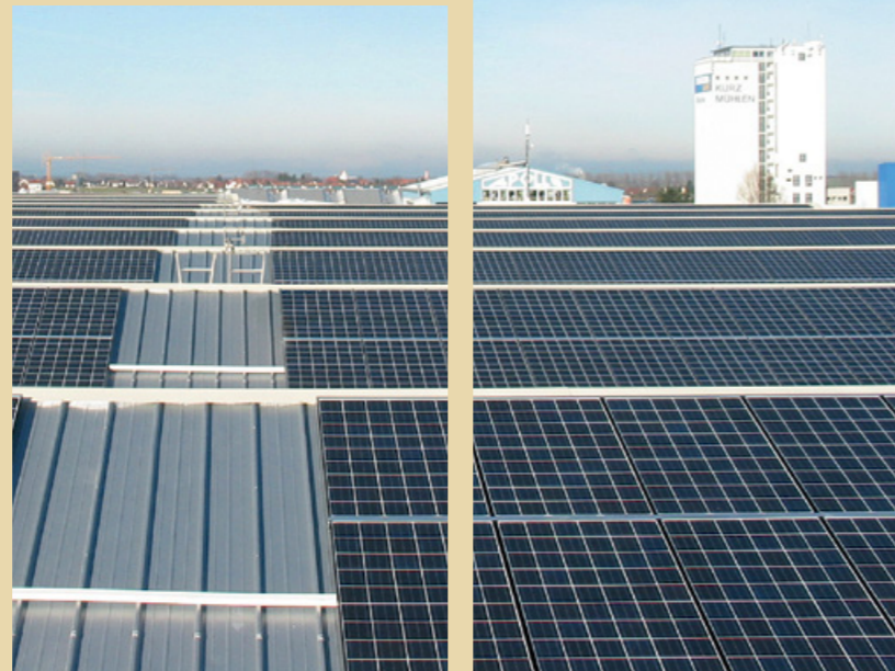
323 kWp, roof-mounted installation, commissioning: 2008
