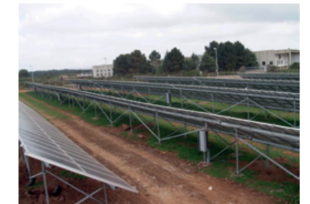
1MWp, ground-mounted installation, commissioning: 2011
