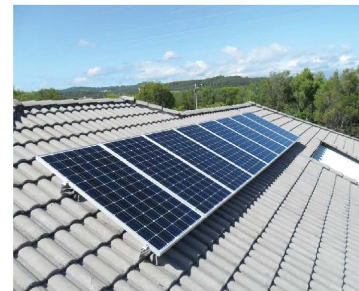
2kW Off-Grid PV
