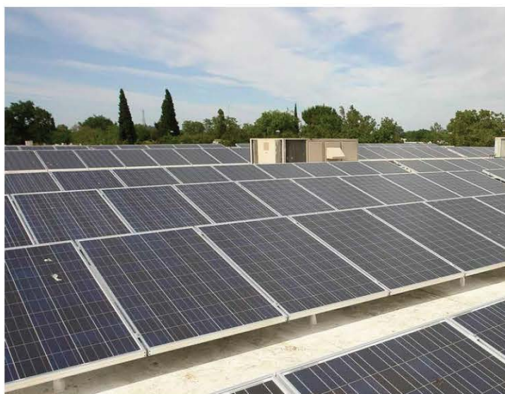
45kWp Flat Roof PV
